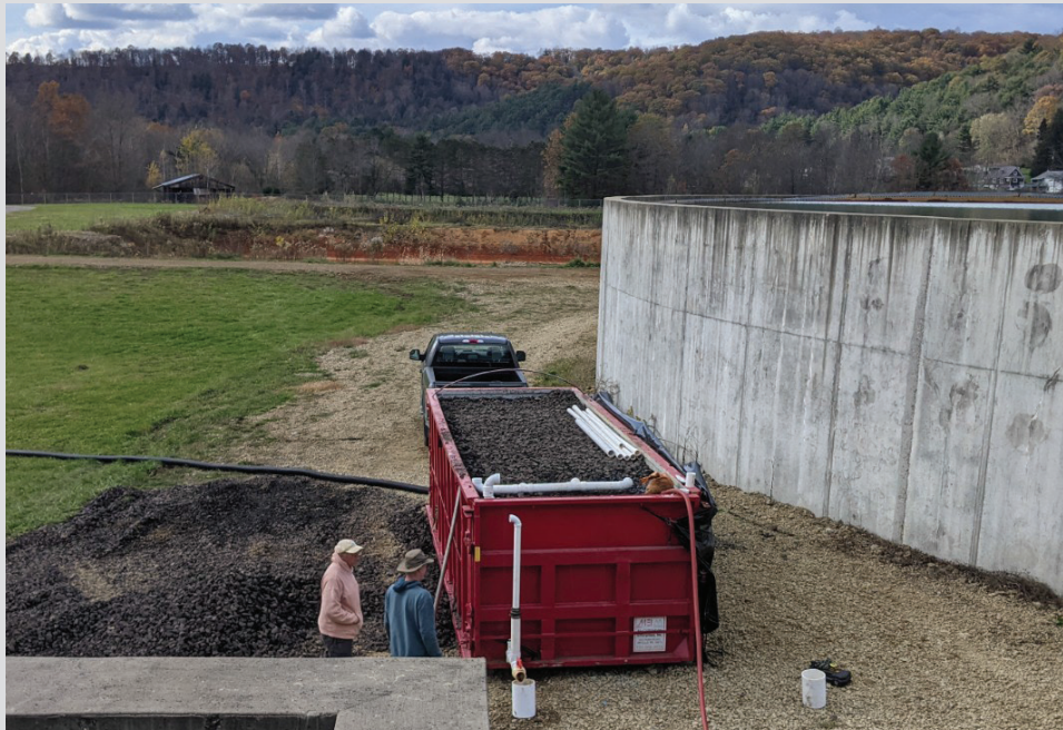
Figure 1 Hollywood pilot scale system in a 23 m 3 roll off container. The Brandy Camp pilot system was similar but an 8 m 3 roll off container
